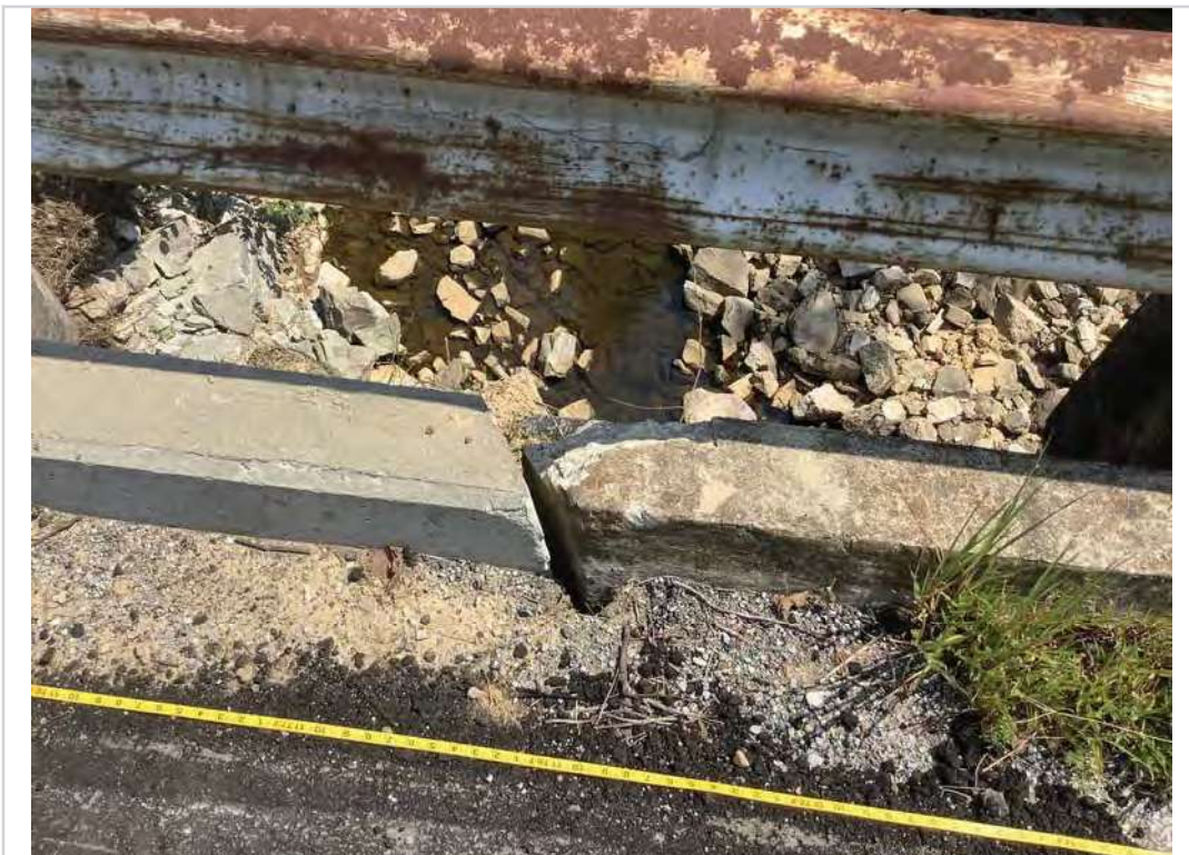
End of span 4 right side curb spalled
