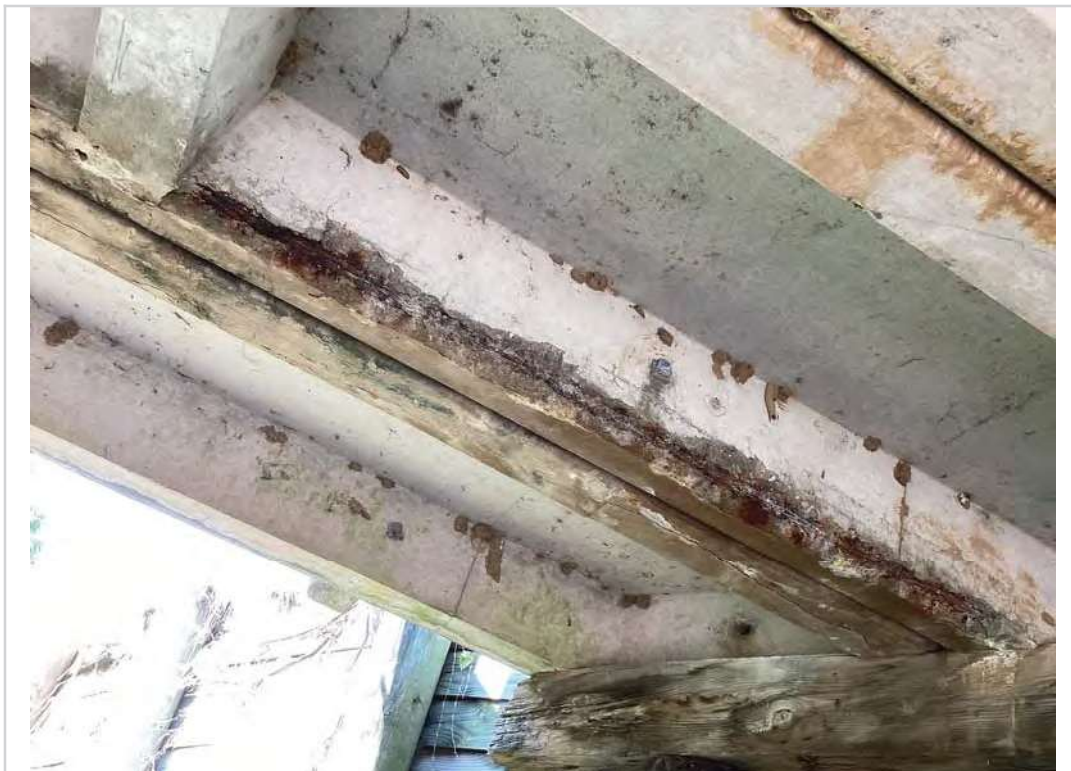
Span #5 PCCS "B" spall to steel
