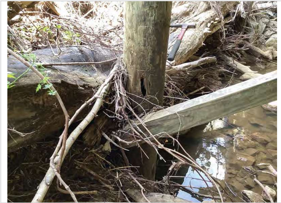
Bent 3 pile A decayed area
