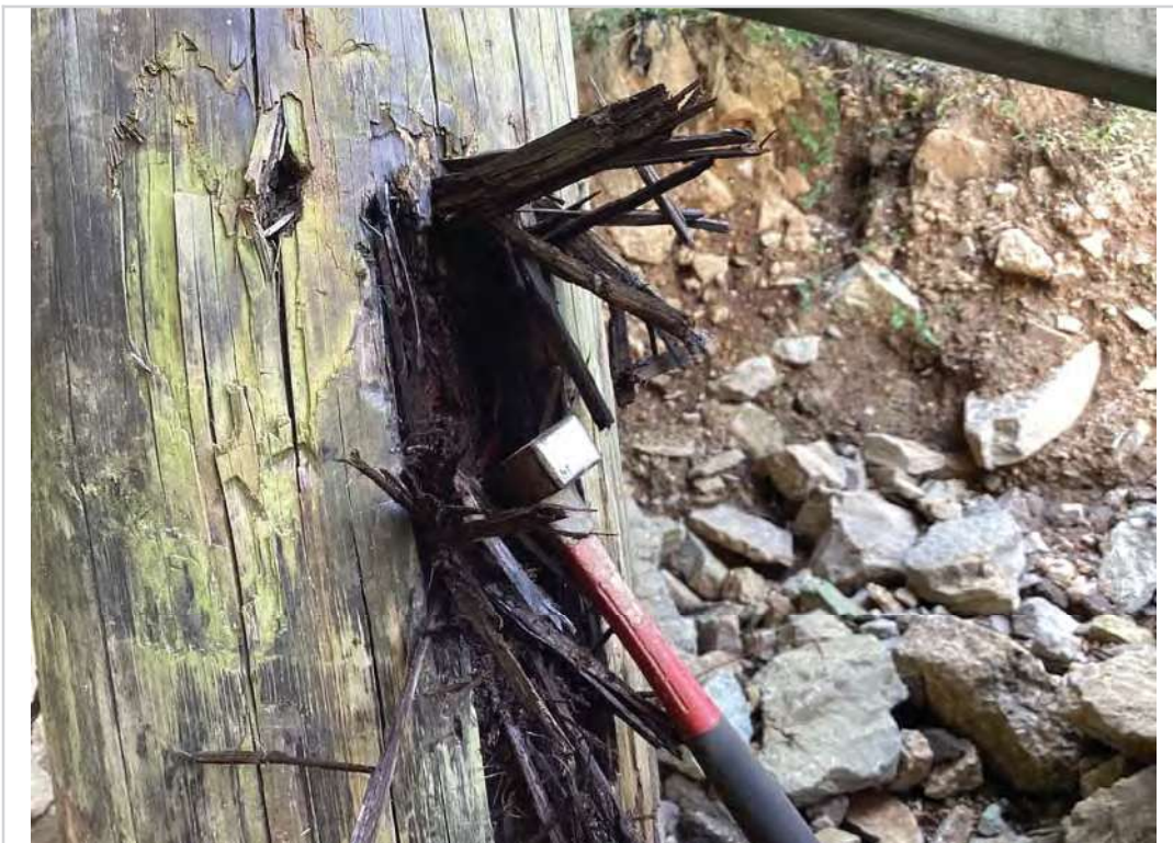
Bent 2 pile B decayed to a 1" shell
