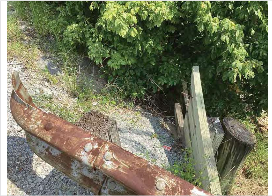
Approach 2 right embankment washing
