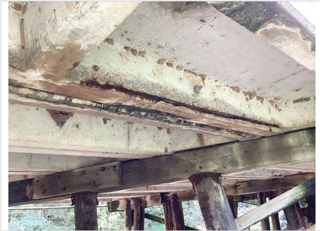
Span #5 PCCS "A" spall to steel
