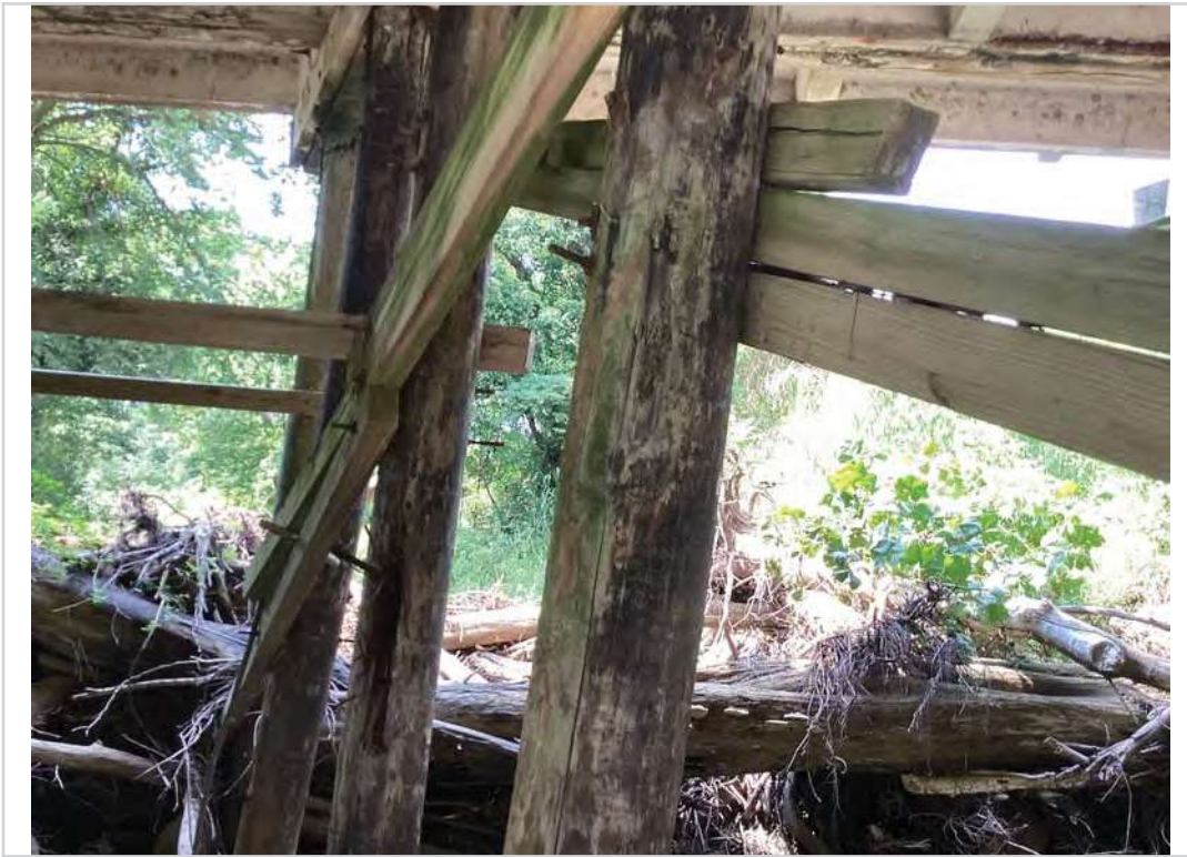
Bent 3 pile D splintered area
