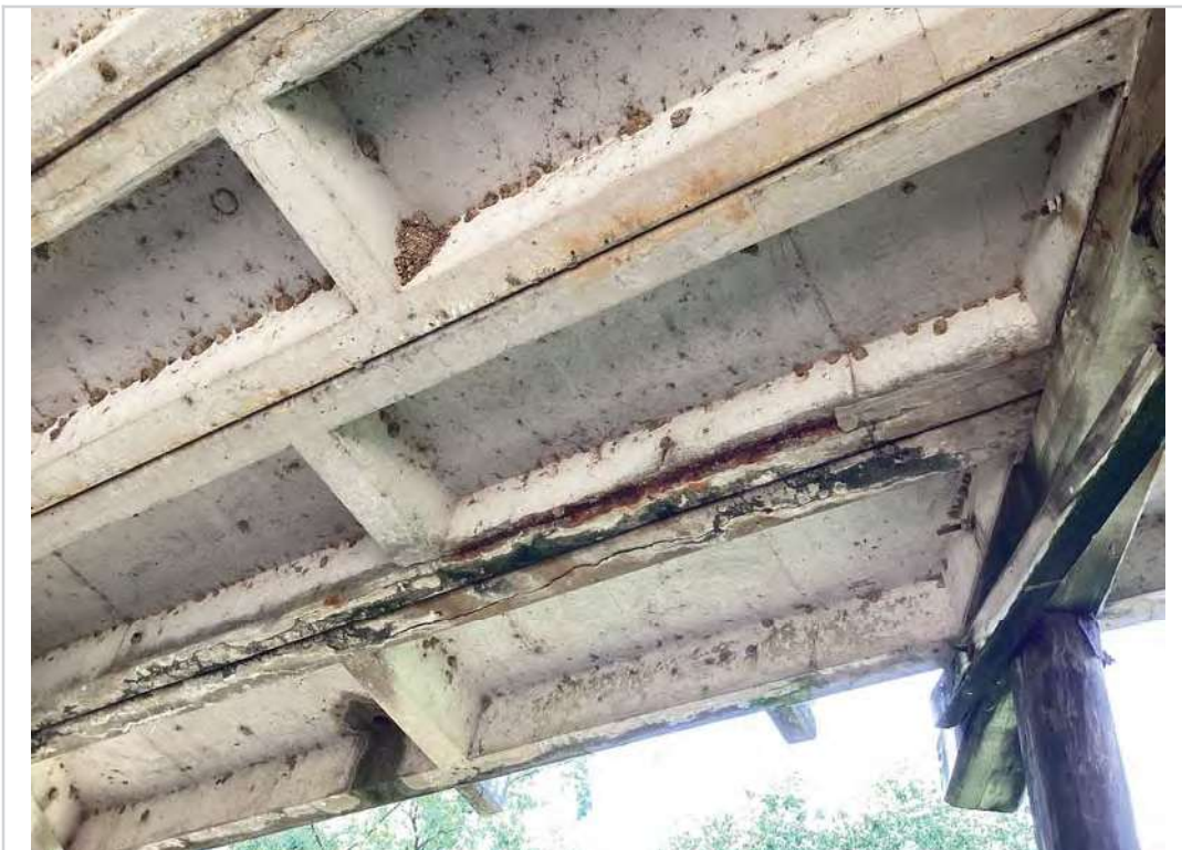
Span #4 PCCS "B" spall to steel
