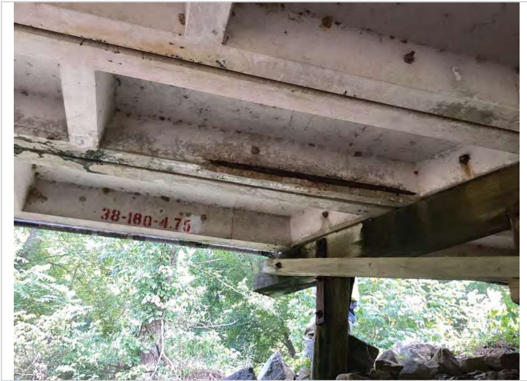
Spall steel slab F span 2
