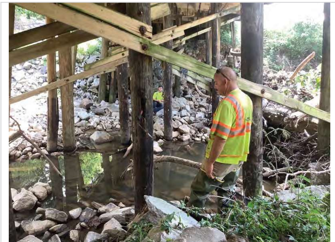
Bent 4 pile C decayed
