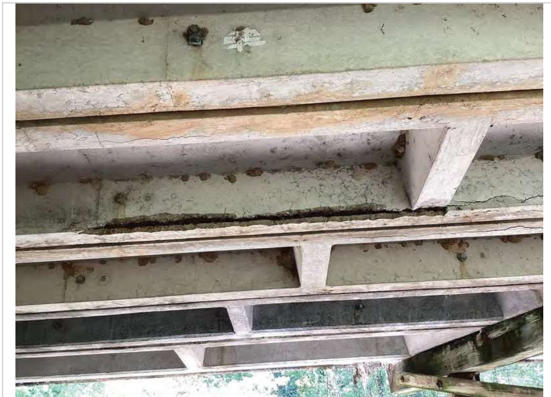
Span #5 PCCS "E" spall to steel
