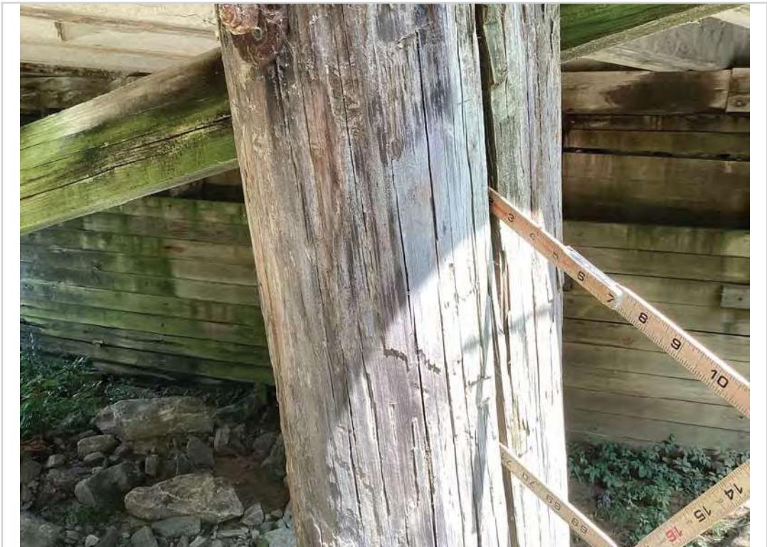
Bent 4 pile f crack 1/4" wide
